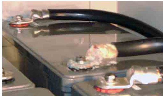
Corrosion on Battery Cable
