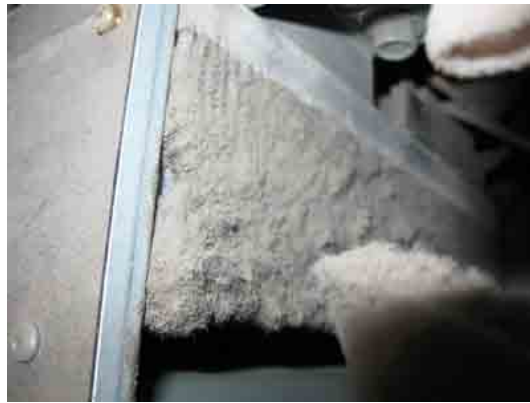
Dust Covered Heat Sink
