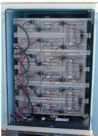
Remote Communications 2 Volt Stack
